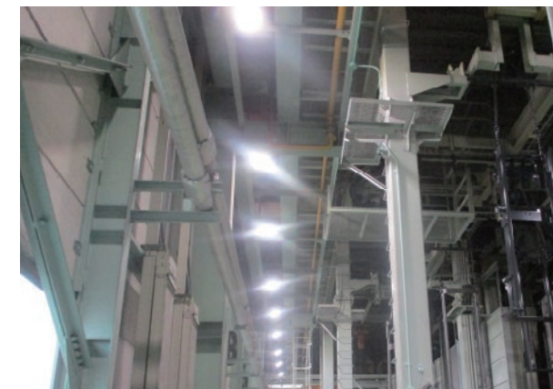
Plant upgraded with new LED lighting fixtures
